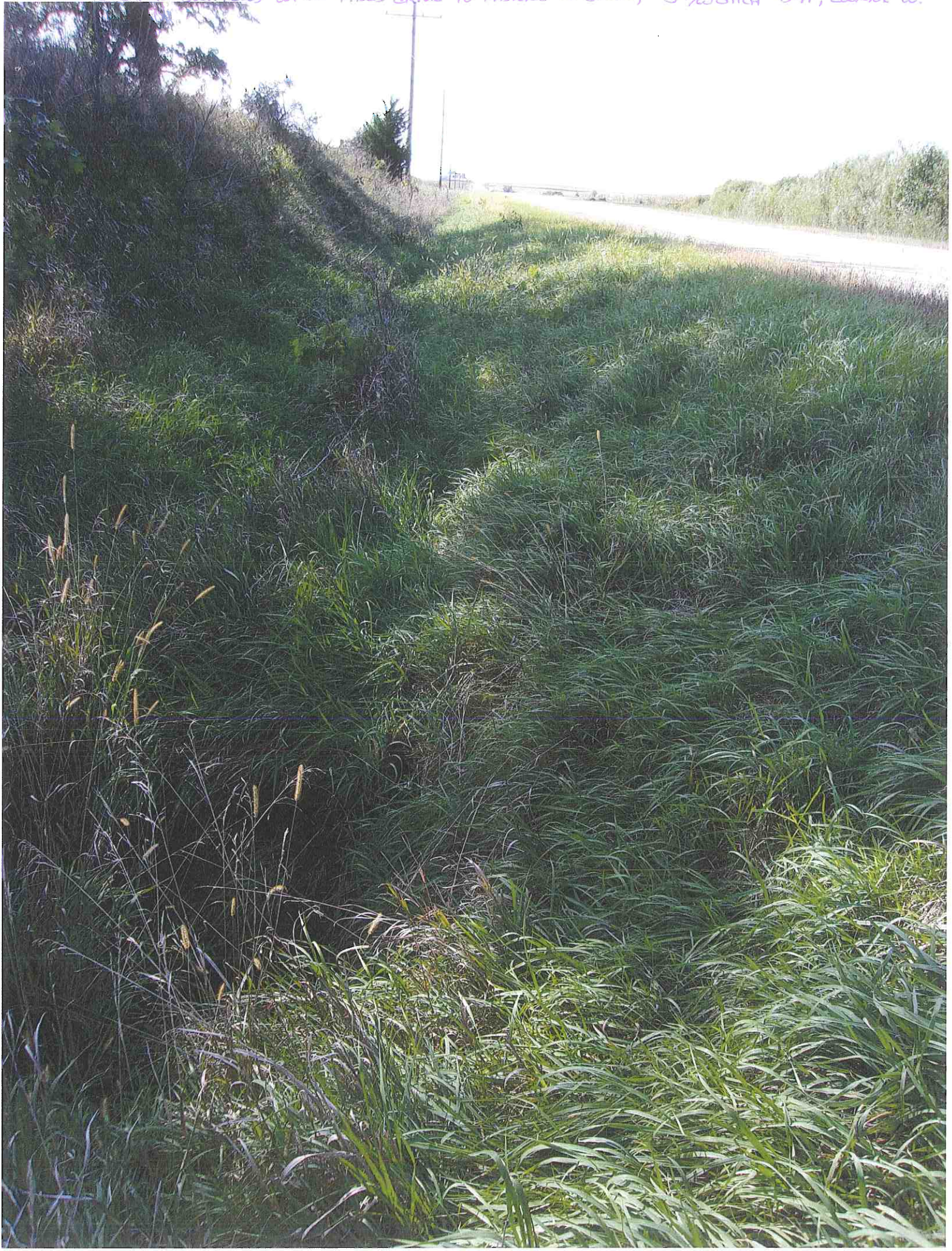
2 LARGE SUCKER PLOWS W. OF FIELD DRIVE TO PASTURE TO SOUTH, S Ditch 041, Location W.
